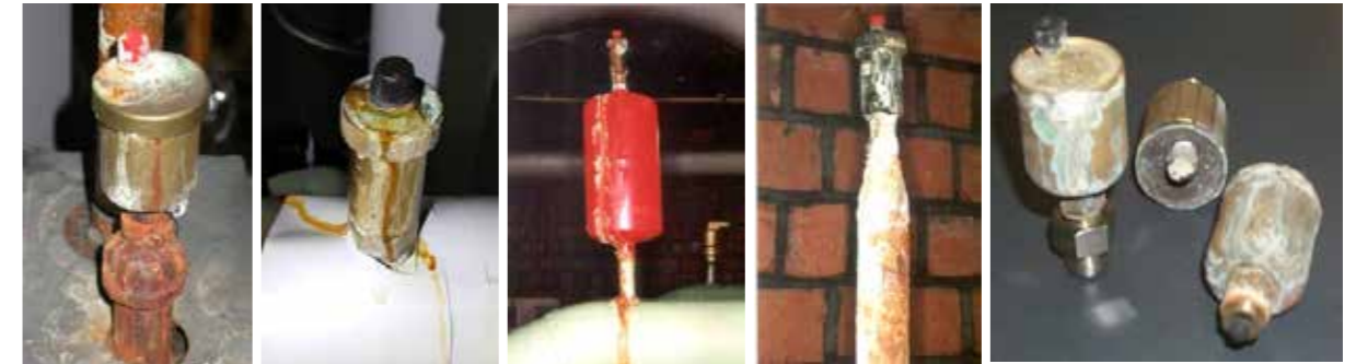
Example of poor-quality air vents, which soon begin to leak due to their faulty construction
